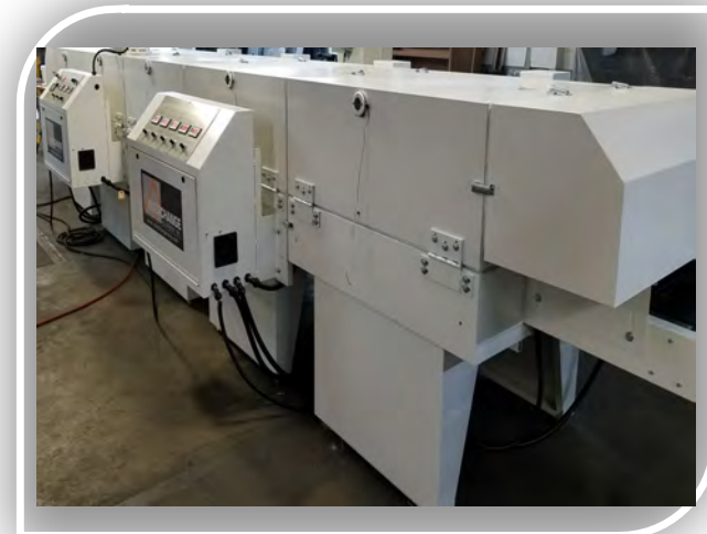
Exit End - With exhaust Hoods
