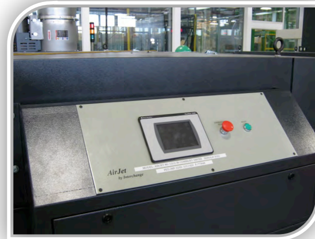
AirJet ALLEN-BRADLEY PLC
